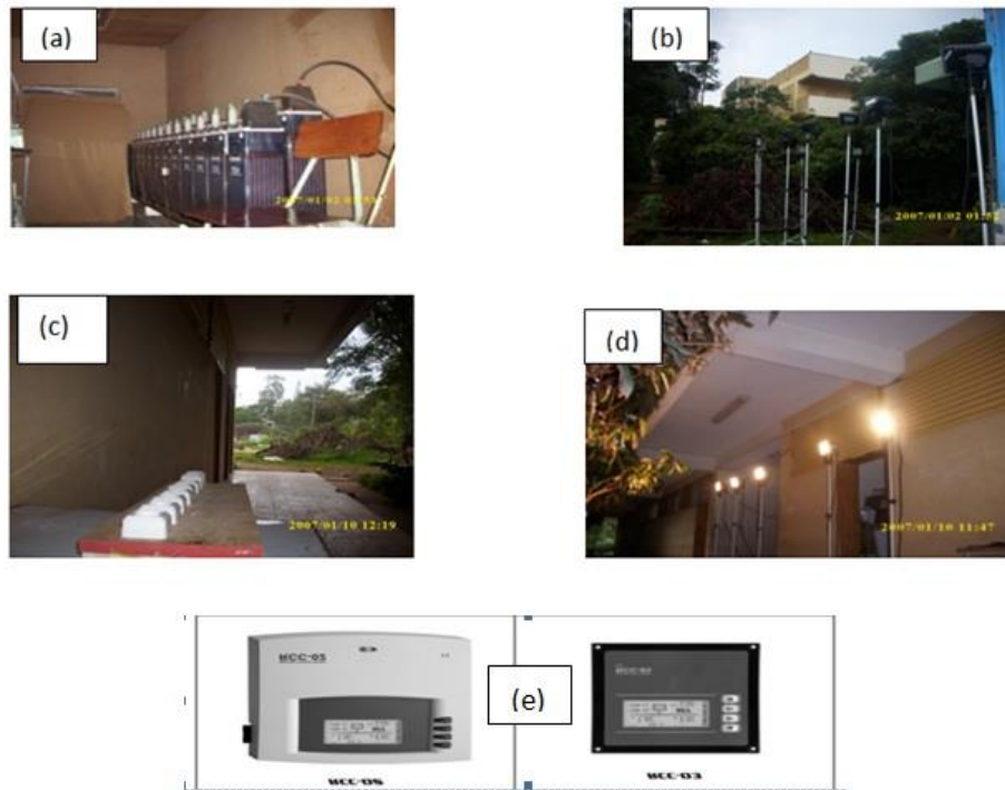
Fig.1: Set up of discharging the battery: a) 24 battery cells in series; b) lamp setup (AC load); c) Divider; d) Lamp lighting by battery power and e) Battery status processor and data Logger unit and SD card
